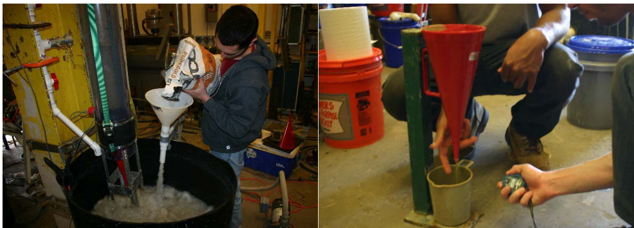
Figure 3.11. Addition of bentonite powder through Hootonanny eductor (left) and viscosity testing of slurry (right)
