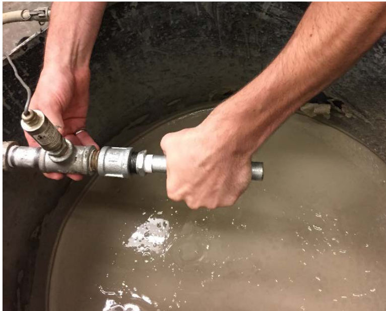
Figure 3.49. Attaching orifice for testing
